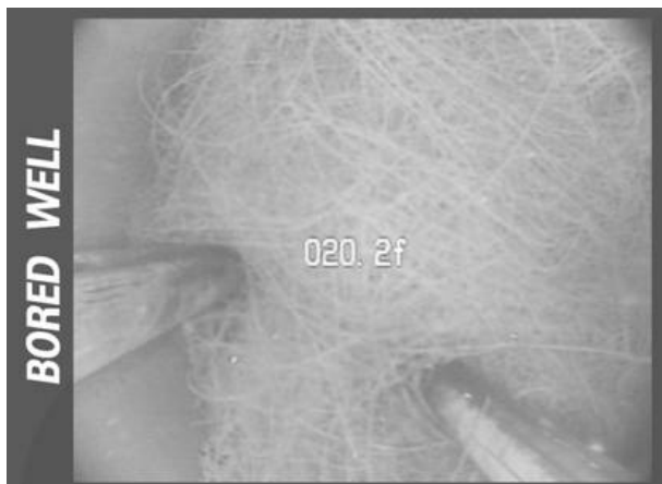
Older wells are more prone to problems, such as roots.
